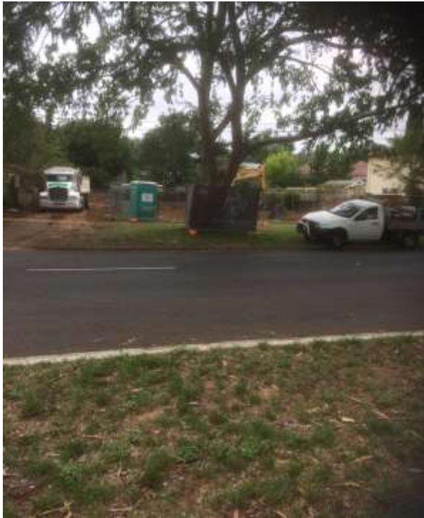
Above: 3 Austin Street, 21 December 2018 at an early stage of construction: but see the next picture below, taken on 5 February 2019.
